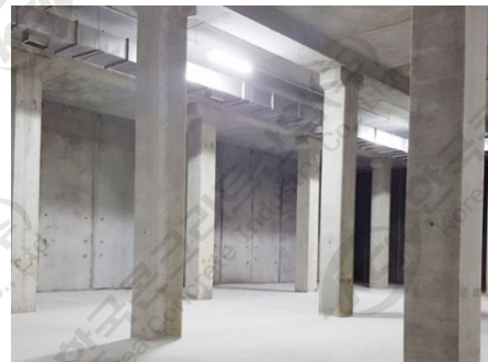
우수저류조 | Rainwater Detention Tank
