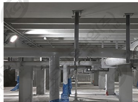
하수·폐수처리장 | Wastewater Treatment Plant
